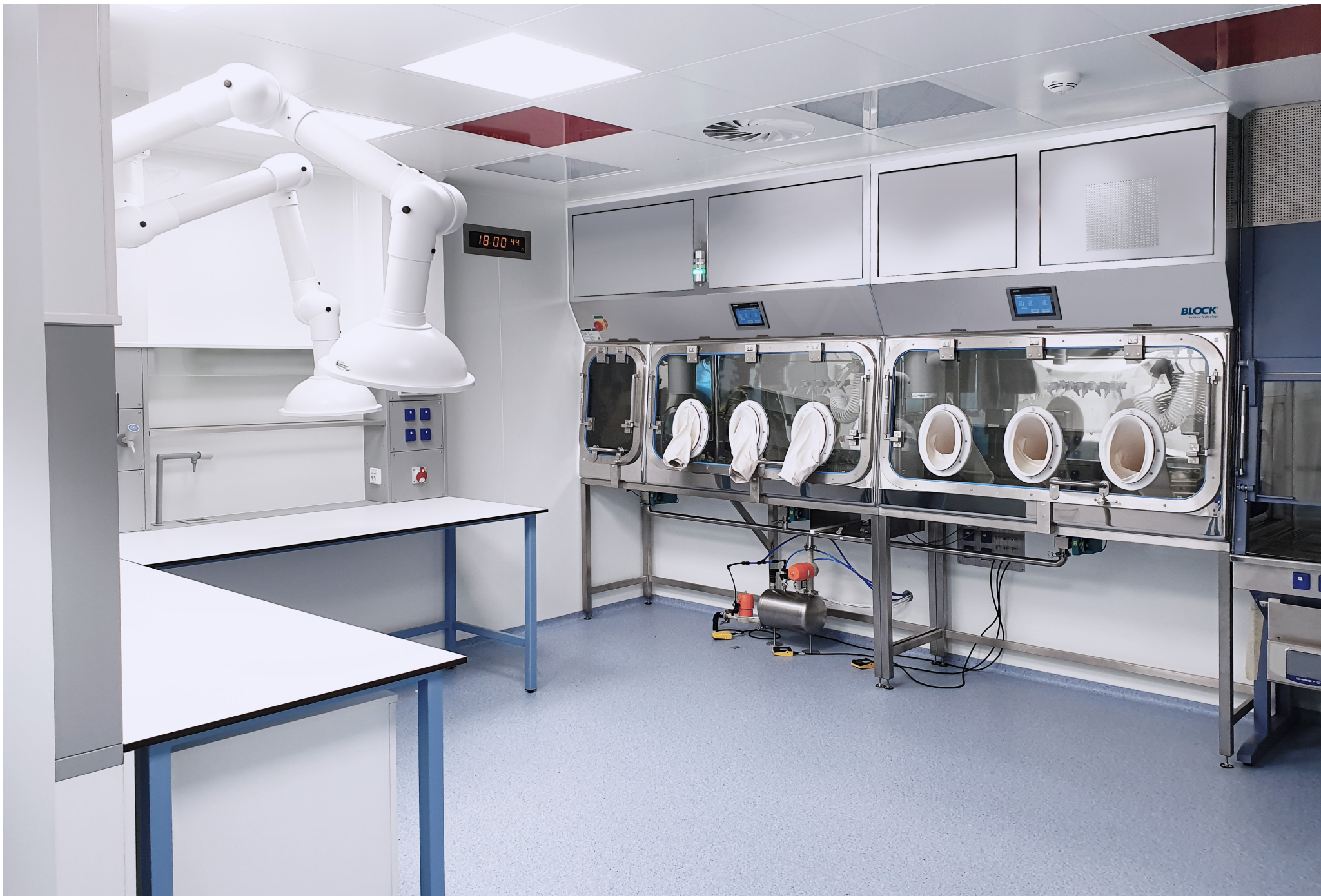
Isolator workplace | Synthon, s.r.o. | Czech Republic
